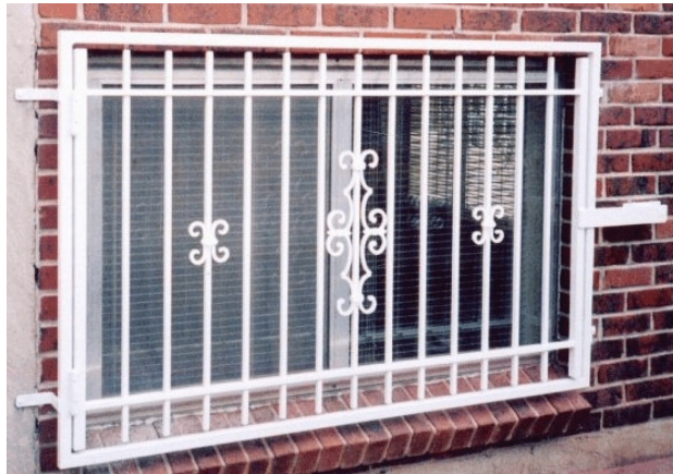
Fire Escape window guards for bedroom windows
